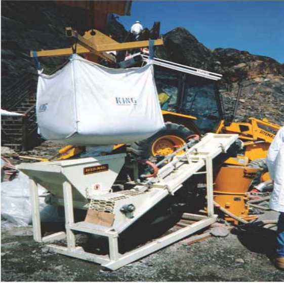
Fig 4: Bagged pre-mix dry shotcrete components being feed to hopper of shotcrete machine.
